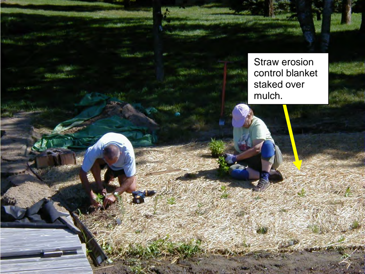
If high water or flooding is possible, a straw erosion control blanket is staked over the mulch prior to planting to prevent the mulch from being washed out. The blanket should have bio-degradable netting . Synthetic photo degradable netting often lasts many years and animals can get caught in the netting.
